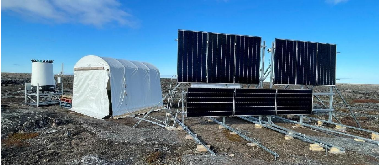
Figure 53: SODAR device (left) along with solar energy array (right) and propane fuel cell station (tent at center).
