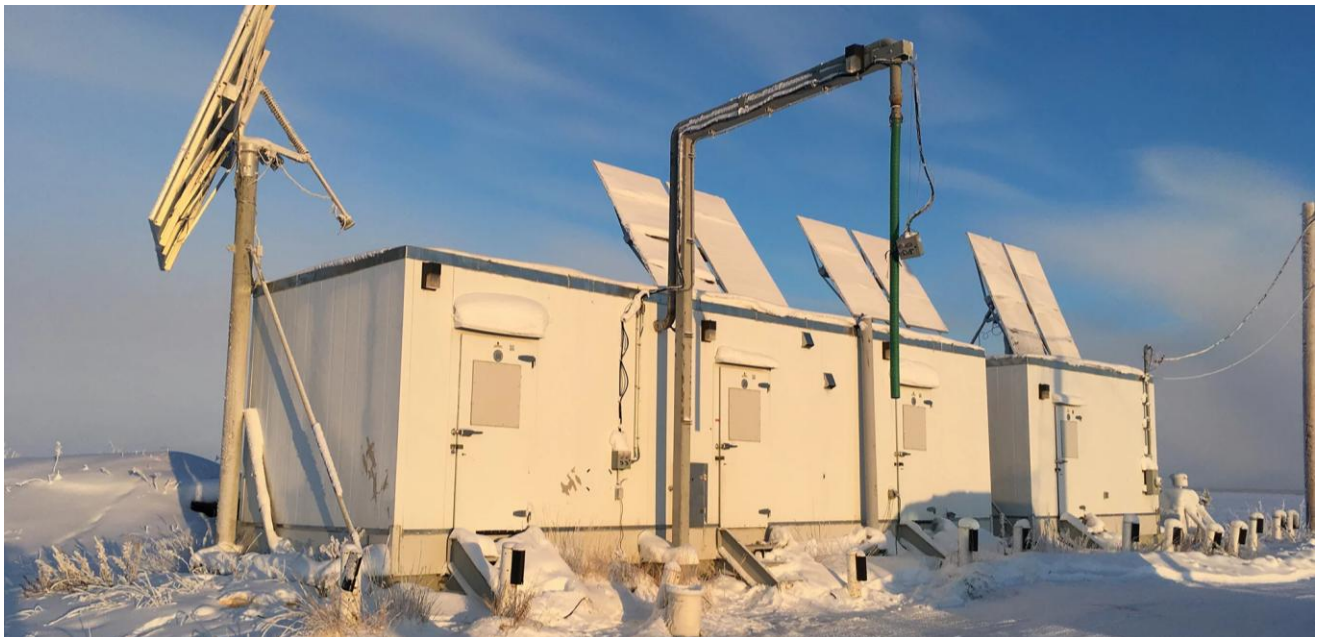
Figure 35: Battery Energy Storage System, Colville Lake, NWT 46
