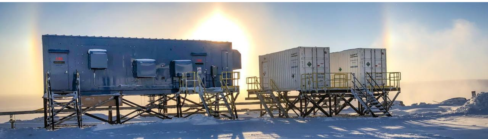
Figure 36: A lithium-ion (Li-ion) energy storage system at Glencore's Raglan Mine, Nunavik, QC 47
