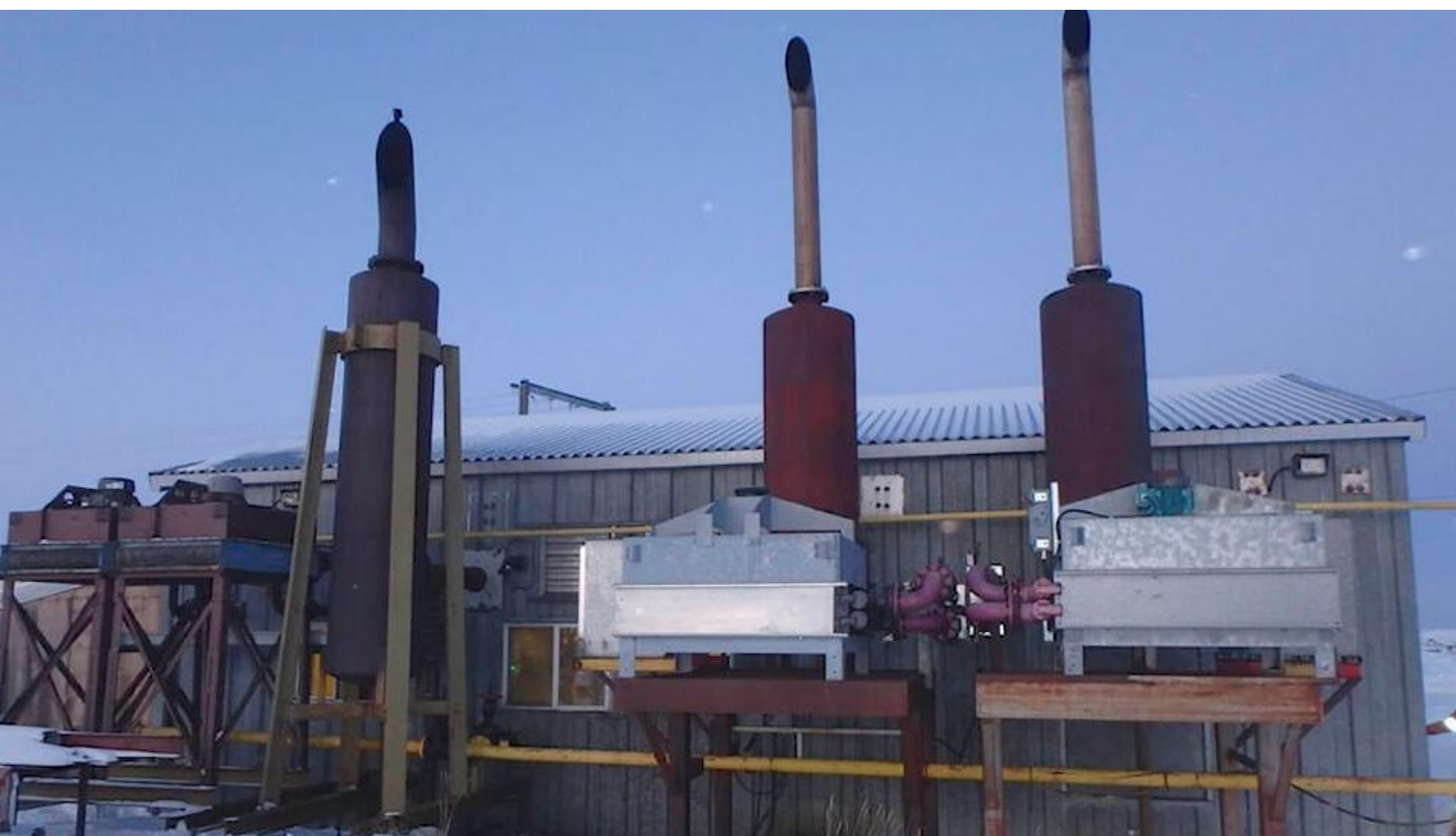
Figure 25: Chesterfield Inlet's current power plant (2022). 30
