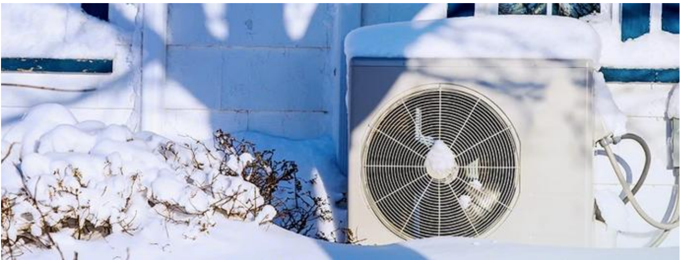
Figure 34: Example of air-source heat pump 40
